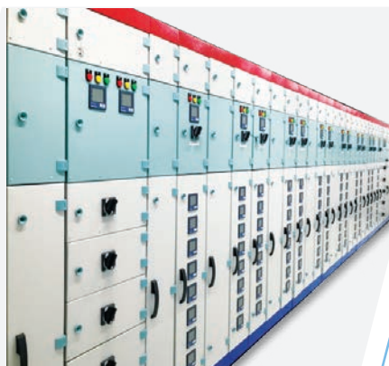
TỦ MBS - DC MBS - DC POWER SWITCHBOARD
